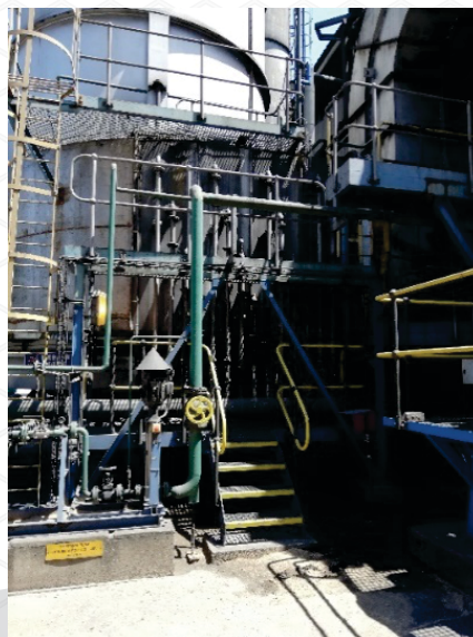
Picture 1. Cyclonic Scrubber Inlet Section
