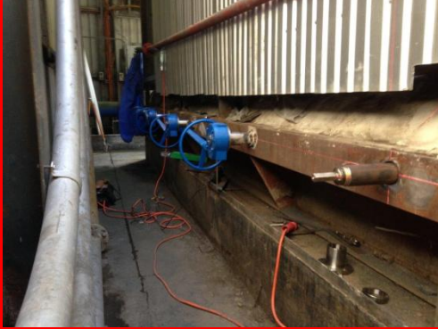
Air Flow Control on a 10 Meg Boiler
