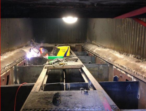
Inside the 10 Meg Boiler
